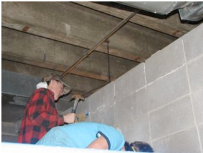
The group from Reddington CC worked to removed two concrete block walls. This is in the basement of Englewood CC where in conjunction with the church, we hope to build a shower room with 3 showers for guys and 3 for girls, each with their own private dressing area. It will be modeled after the MI shower trailer, and will be used when the weather is too cold for the shower trailer.
