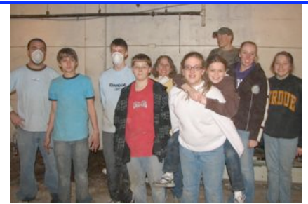
The Reddington group standing where walls had been six (6) hours earlier. The best part is that they were able to save about 90% of the cement blocks for use on future projects.
