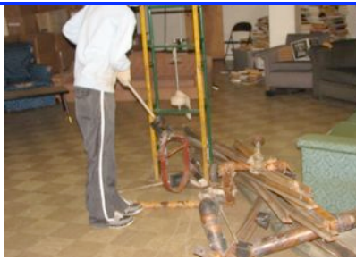
In addition to the block walls, there was a lot of pipe and miscellaneous scrap to remove.
